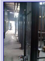
Construction is progressing on the interior of the new PET / CT suite at CCA Lake Hefner.
